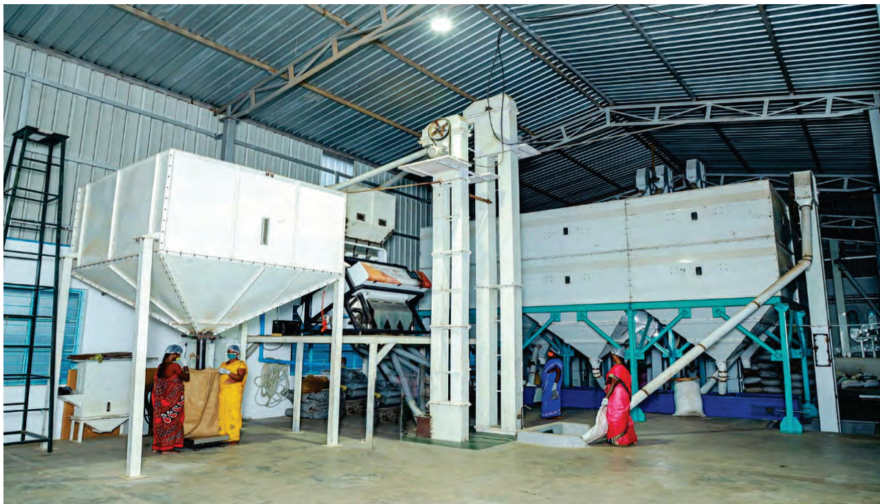
A Coffee Beans Processing unit assisted under NEED Scheme, Dindigul District
