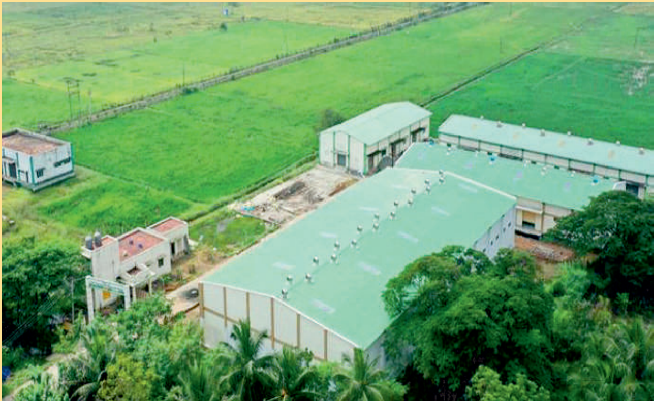
Construction of Regulated Market at Poonthottam with warehouse capacity of 2000 MT and 1000 MT.
