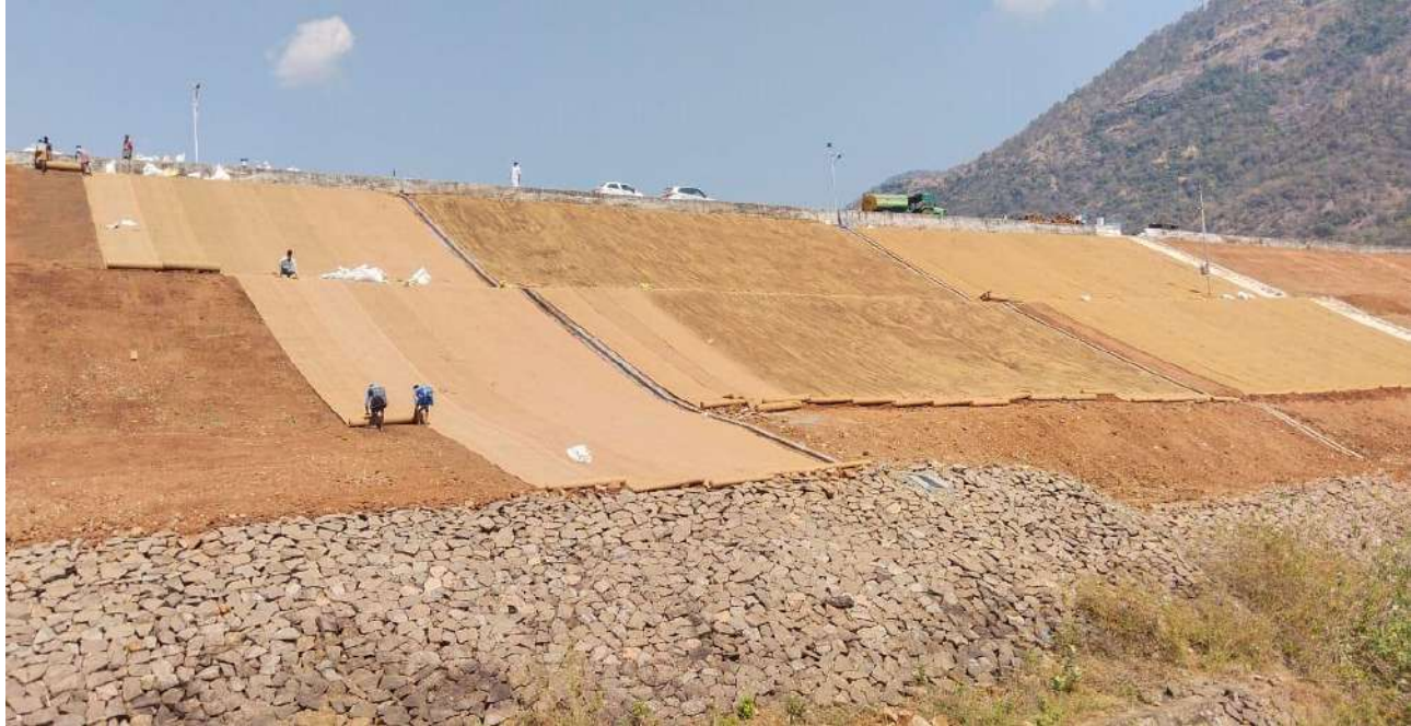
Theni District -Installing Coir Geo-textiles for Erosion Control on the sloping (rear) side of Manjalar Reservoir - Estimate Rs.2.09 crore - State Fund
