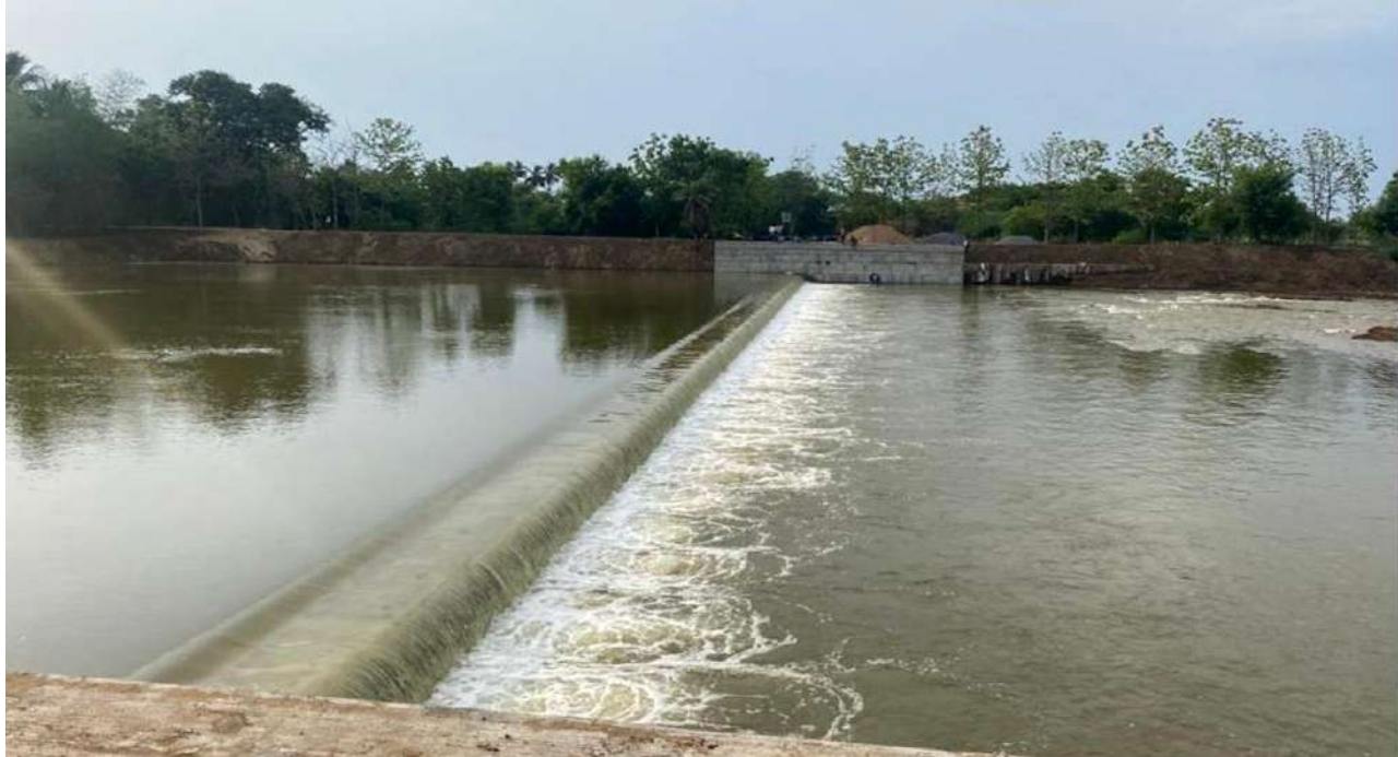
Thanjavur District - Grade wall across Vettar River at LS 73.635 Km in Surakkayur village - (Estimate Rs.4.88 crore) - NABARD
