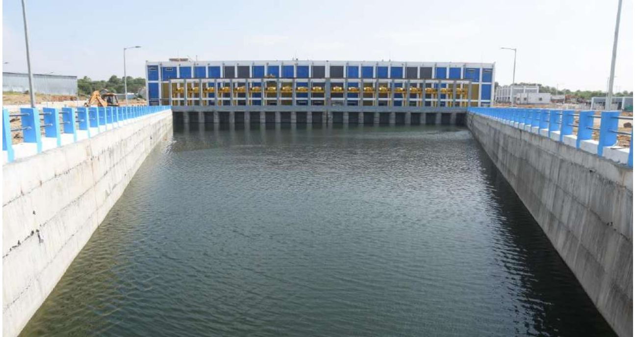
Salem District - Mettur Sarabanga Lift Irrigation Project Thippampatti Pumping Station – (Estimate Rs. 565.00 crore) – State Fund
