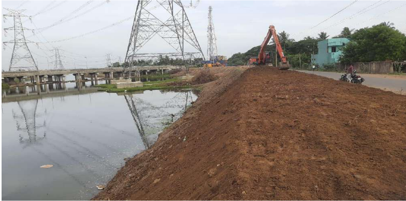
Thiruvallur and Chennai District- Restoration and Reformation of River Bund and regradation of River Bed in Kosasthalaiyar River - Estimate Amount Rs. 15.00 crore - State Fund
