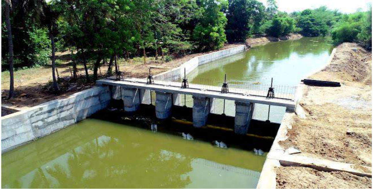
Mayiladuthurai, Thanjavur & Thiruvarur District- Extension, Renovation and Modernisation -Cauvery subbasin- Regulator across Keerthimannar River (Package No -21) – (Estimate Amount Rs.136.54 crore) - NIDA
