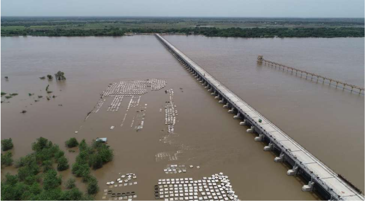
Cuddalore & Mayiladuthurai Districts- Construction of Barrage across River Coleroon in between Adhanur and Kumaramangalam villages - (Estimate Rs. 494.60 crore) – State Fund
