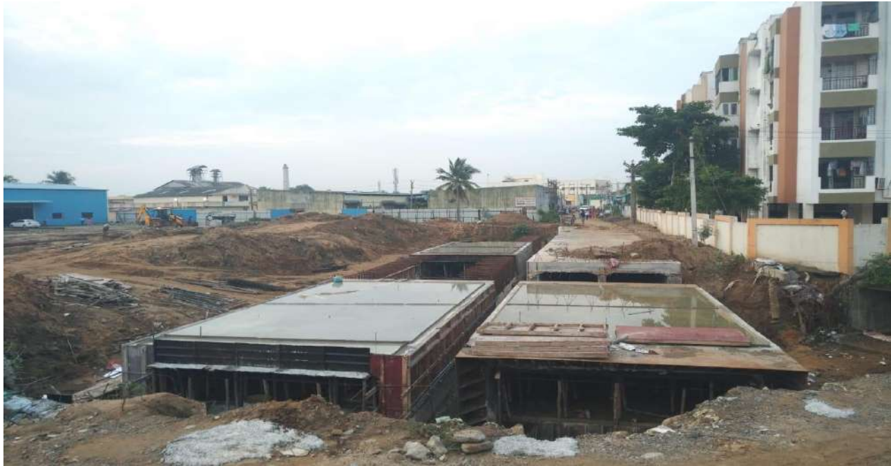
Kancheepuram District- Providing additional Box culverts at NH Bypass - Estimate Amount Rs. 9.70 crore- State Fund
