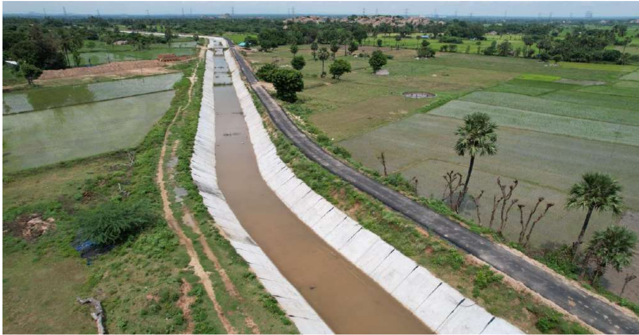
Villupuram District - Improvements to Nandhan Channel From LS12.400 Km to LS 37.880 Km in Gingee, Vikkravandi and Villupuram Taluks - Estimate Amount Rs. 26.57crore - NABARD
