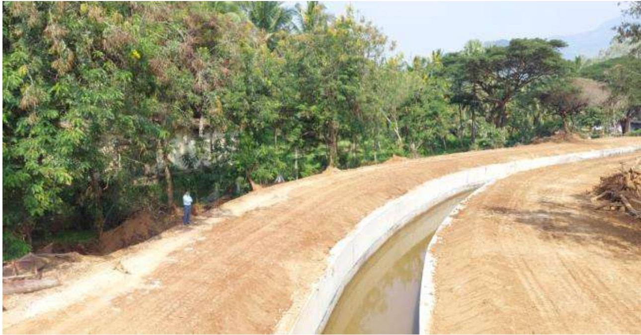
Coimbatore District - Anaimalai Taluk, Rehabilitation of Pollachi Canal without lining of canal and bed from LS 0/000 Km to 20/000 Km and its distributaries - Estimate Rs.4.09 Crore - NABARD Fund
