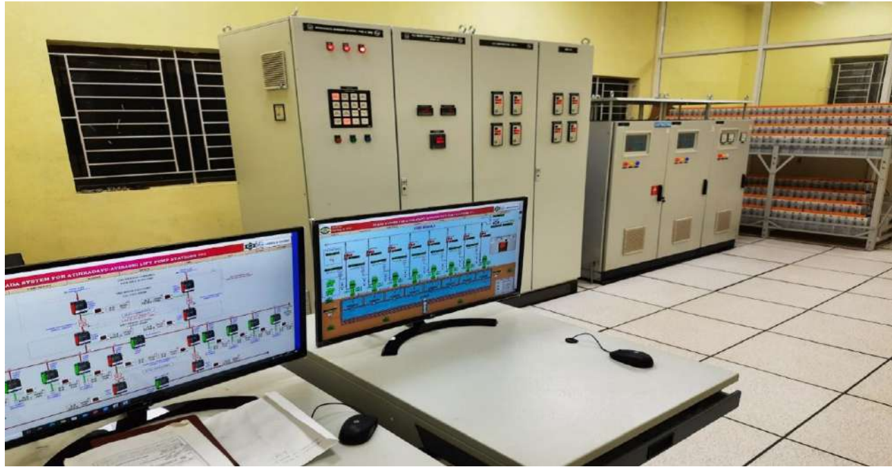
Erode District – Bhavani Taluk, Athikadavu Avinashi Pumping Scheme, Automated Control Room (SCADA) at Bhavani– Estimate Amount Rs.1756.88 Crore – State Fund
