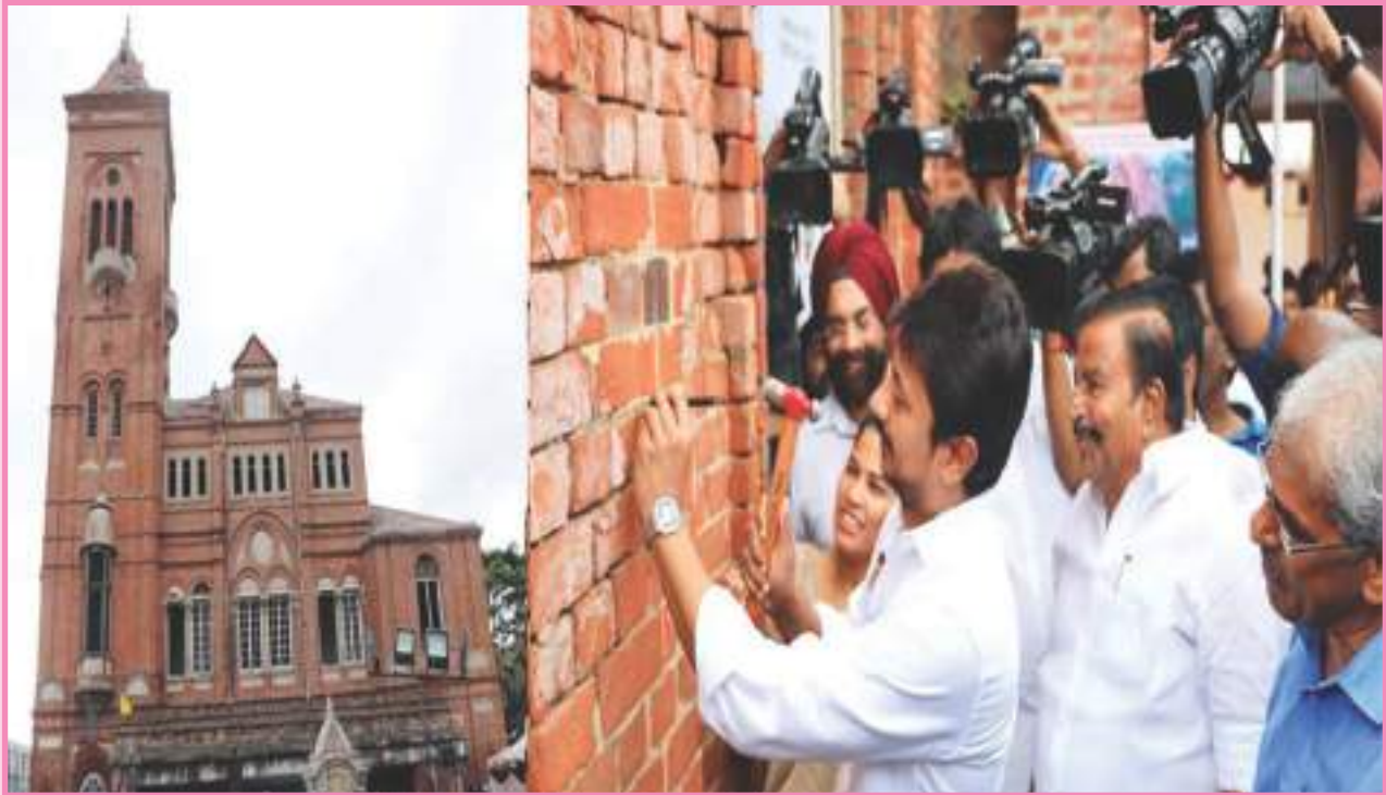
Conservation, Revitalization and Retrofitting work of the Victoria Public Hall in Chennai, under Singara Chennai 2.0 at a cost of Rs. 32.62 crore commenced on 20.03.2023
