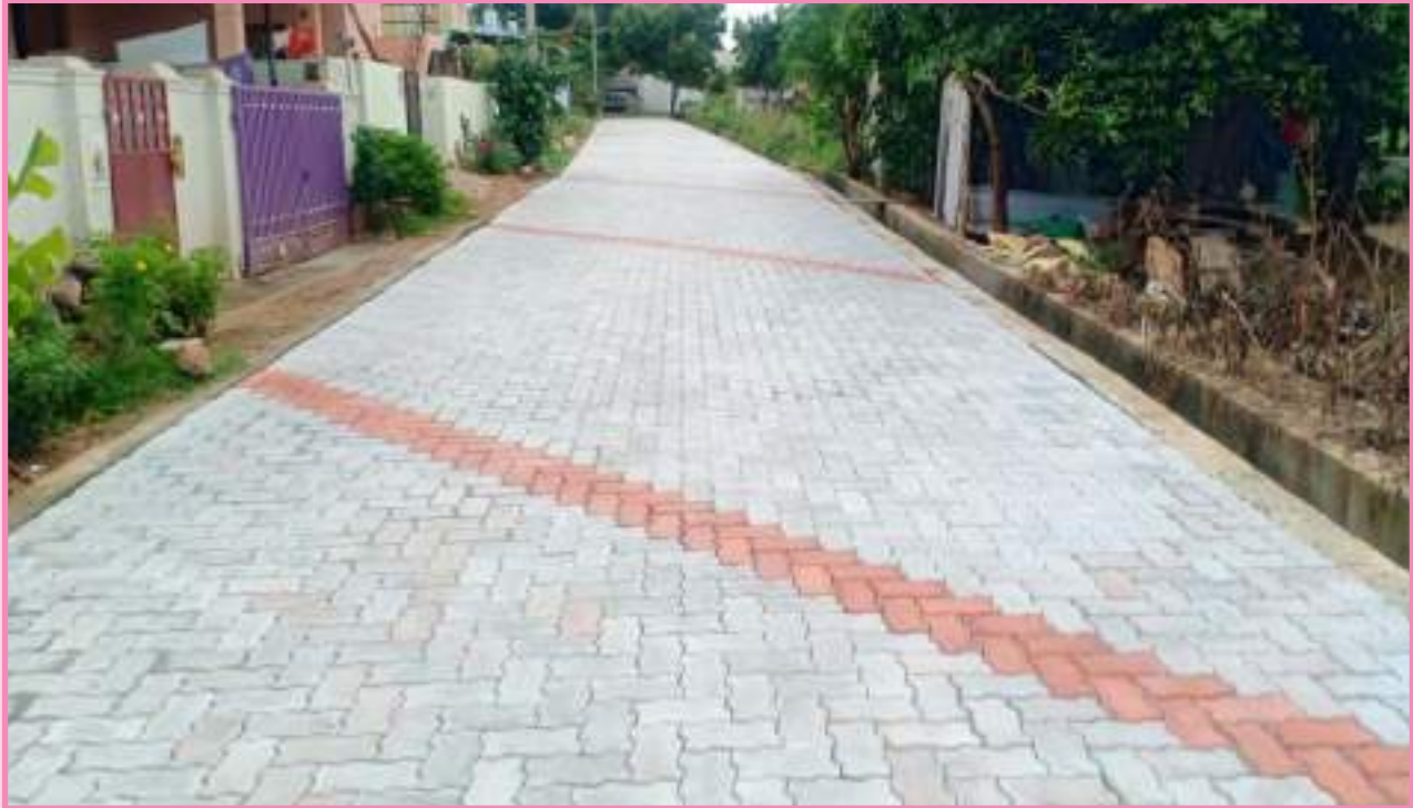
Construction of paver block road and stormwater drain at Sri Sampathkumar Nagar, Odayakulam town panchayat (Coimbatore district), Scheme : Kalaingar Nagarpura Mempoattu Thittam; Project cost : Rs. 52.78 lakh
