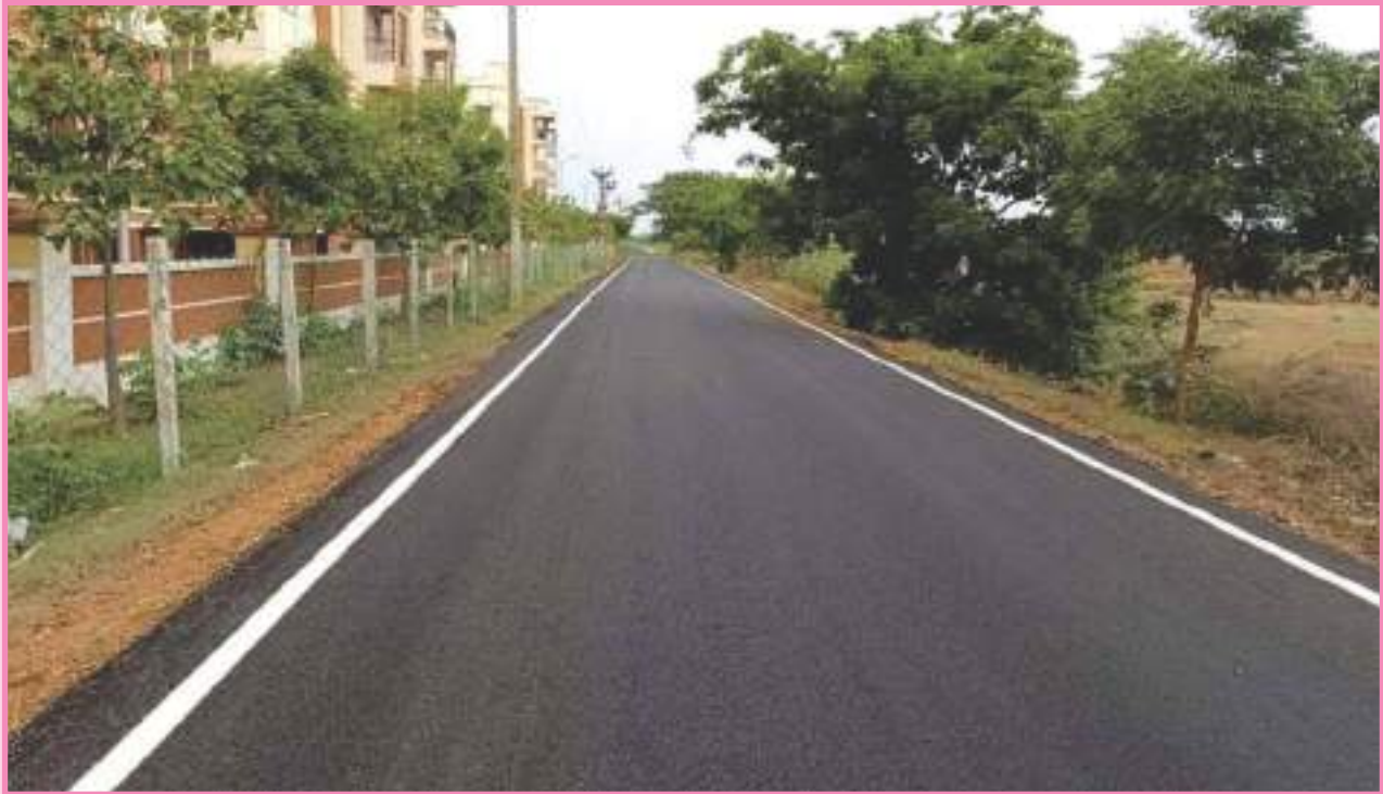
Construction of a new BT road (earthen road to BT road) in Thiruporur town panchayat (Chengalpattu district), Scheme : Capital Grant Fund; Project cost : Rs. 1.00 crore
