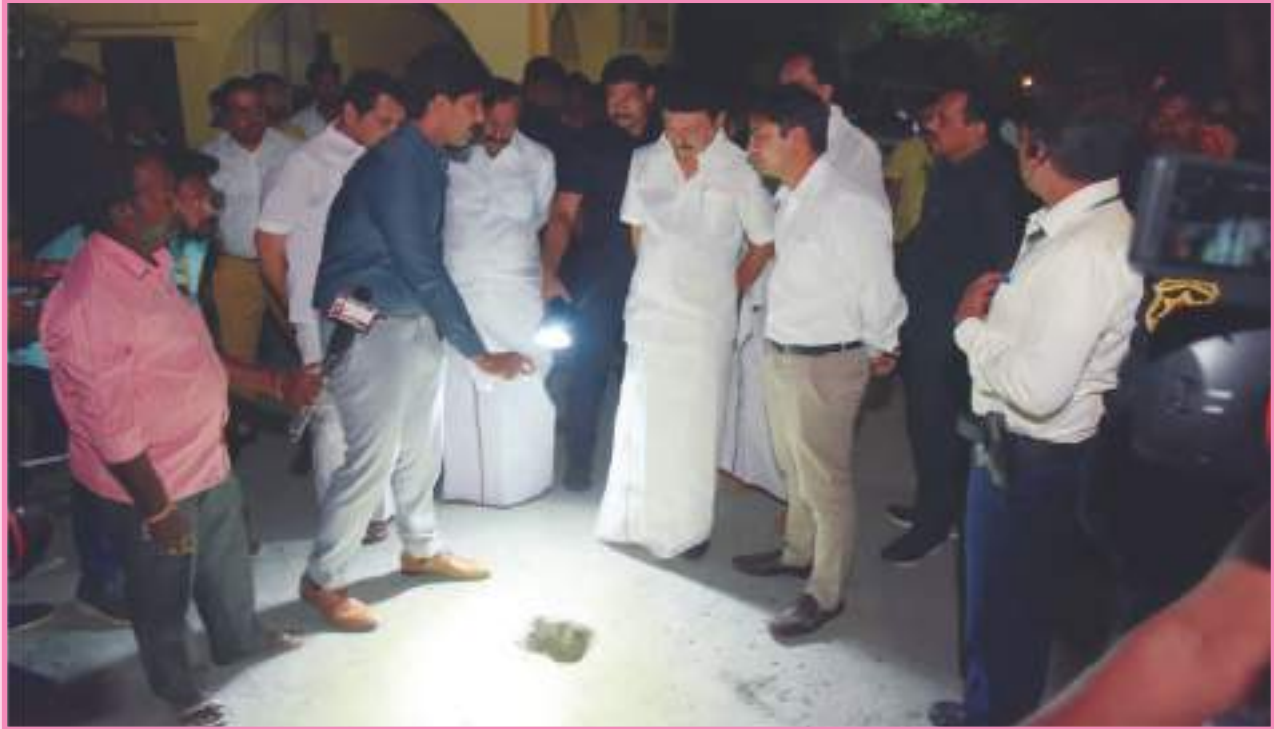
Honourable Chief Minister inspecting the quality of the road laid at PSG HUDCO colony at Peelamedu, Coimbatore
