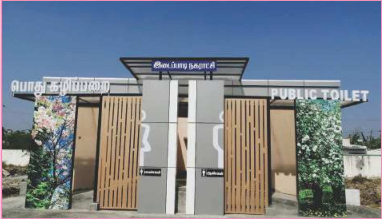
Construction of public toilet at Vellandivalasu in Idappadi municipality (Salem district), Scheme : Swachh Bharath Mission 2.0; Project cost : Rs. 36.28 lakh
