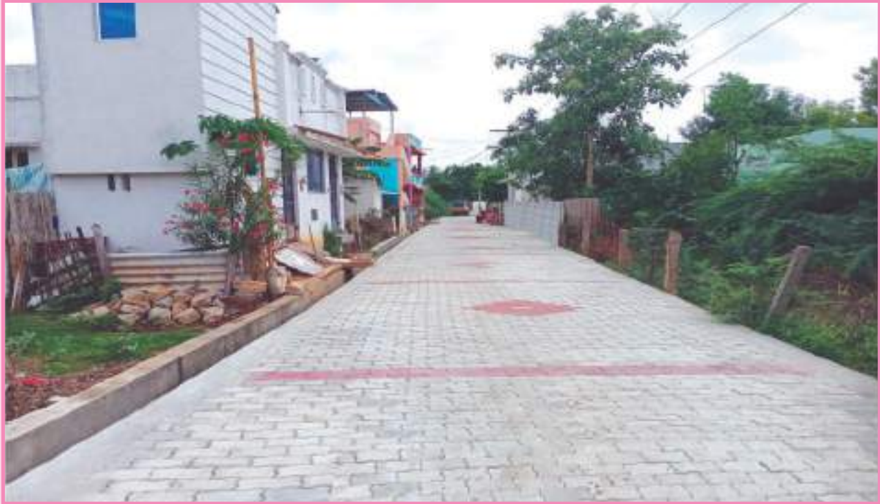
Construction of paver block pavement and stormwater drain in Thuvakudi municipality (Tiruchirapalli district), Scheme : Kalaignar Nagarapura Mempattu Thittam; Project cost : Rs. 28.70 lakh
