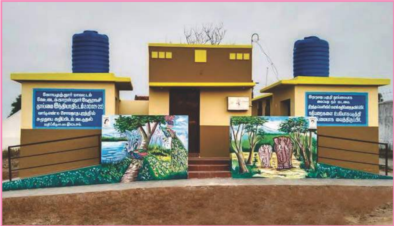
Construction of community toilet in Vettaikaran Pudhur town panchayat (Coimbatore district), Scheme : Swachh Bharath Mission 2.0; Project cost : Rs. 15.00 lakh
