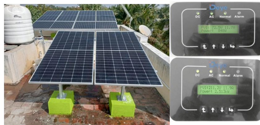
(3+1) kW Rooftop Solar PV System installed at Madurai under GCRTS – Phase II
