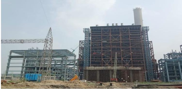
Turbo Generator Unit I
