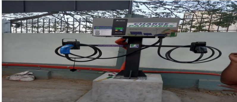
25 kW Solar Powered EV Charging Station, DPI Complex, Chennai
