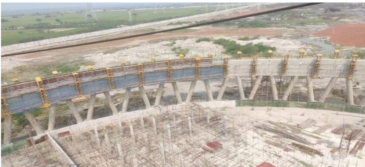
Natural Draught Cooling Tower 1
