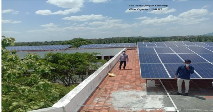
300 kW Rooftop Solar PV system at Periyar University
