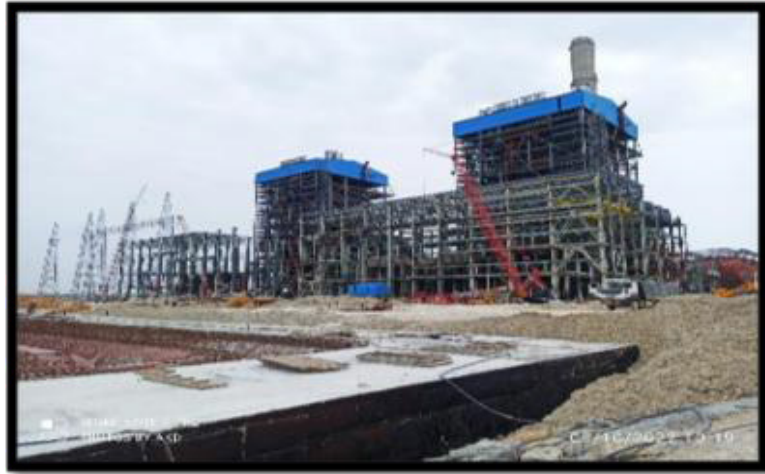
MAIN PLANT VIEW
