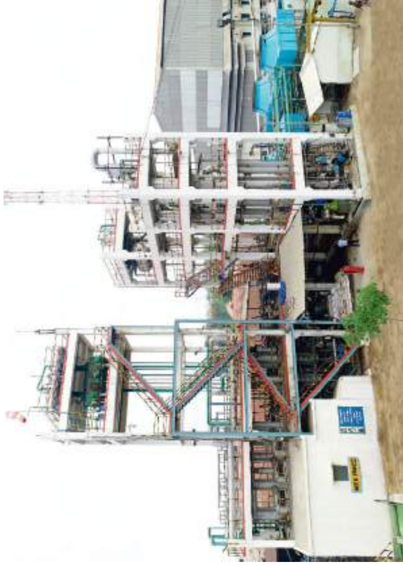
Multiple Effect Evaporator with Crystallizer in Textile CETP at Tiruppur
