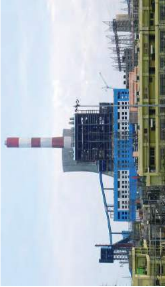
North Chennai Thermal Power Projects Stage-III
