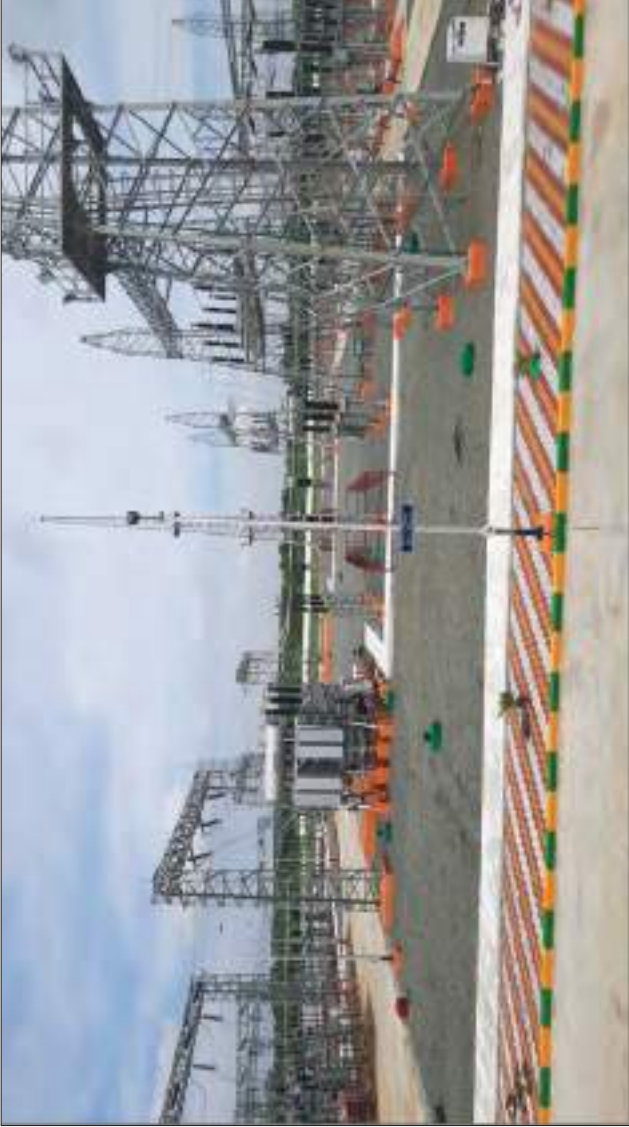
Thuvakudy 230 kV SS - Trichy District
