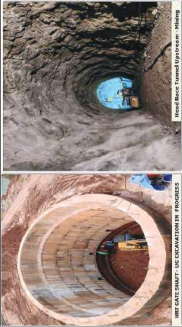
Kundah Pumped Storage Hydro Electric Project
