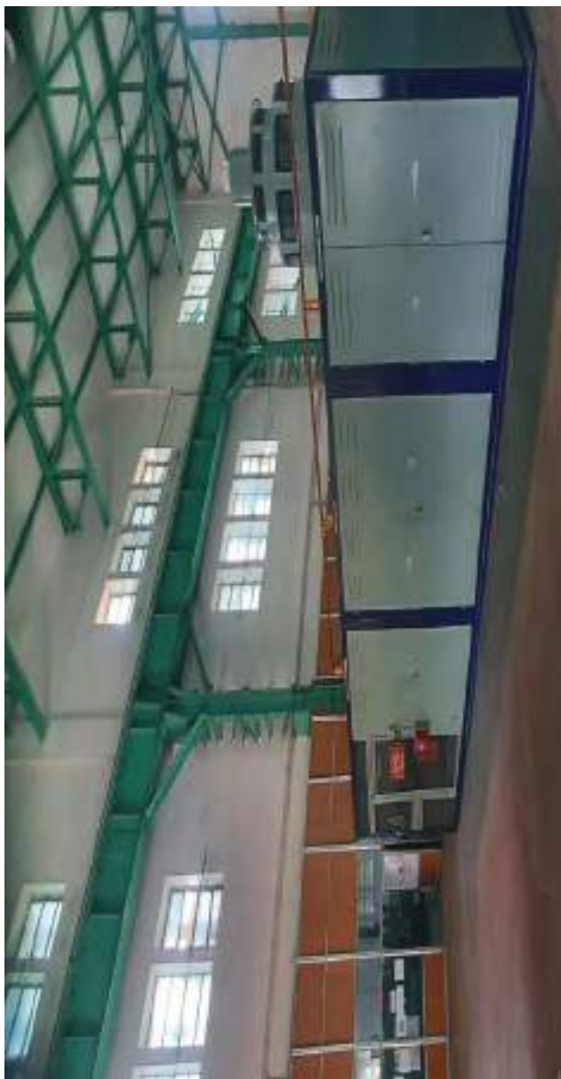
Aliyar Power House
