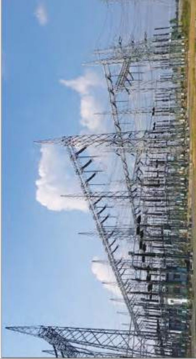
Ariyalur 765 kV AIS - Kallakurichi District
