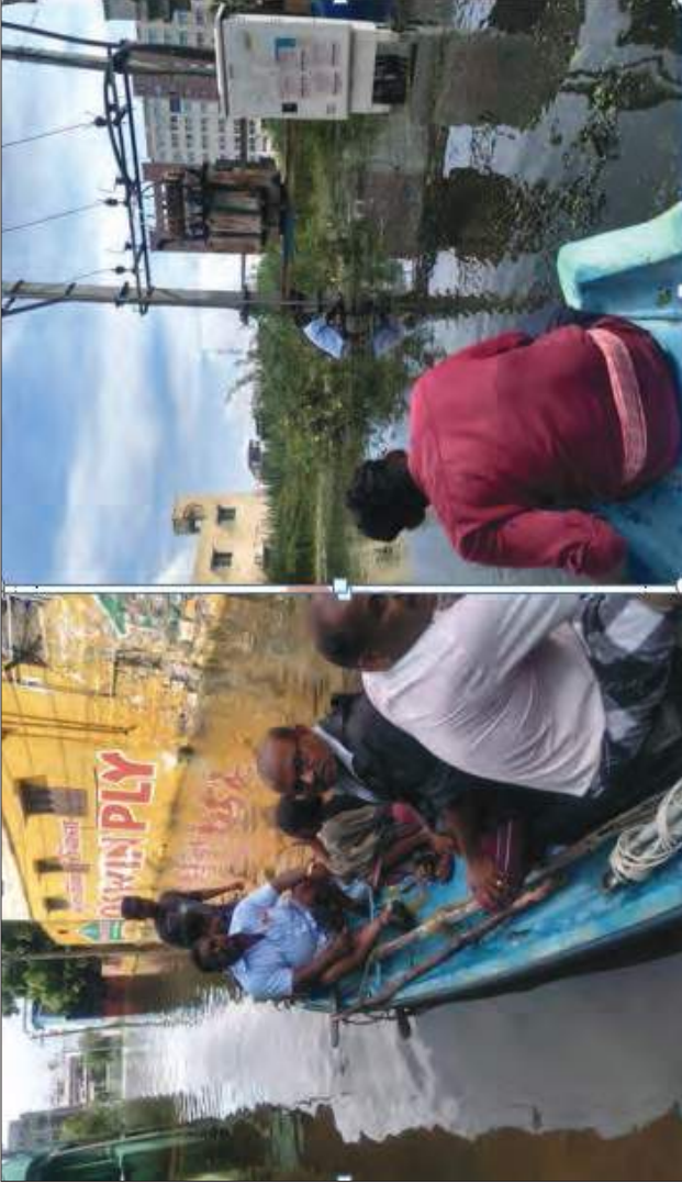
Distribution Transformer charging at Madhavaram II section / Chennai North EDC
