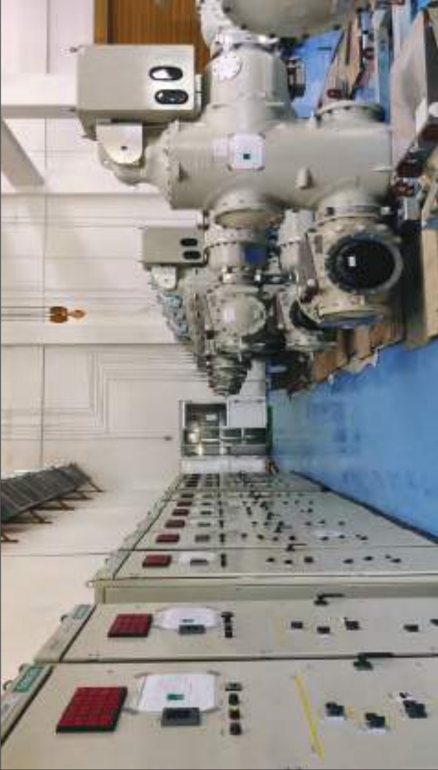
Erode 230 KV GIS – Erode District
