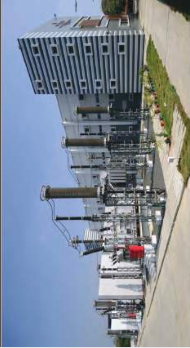
Guindy 400 kV GIS - JICA Chennai District
